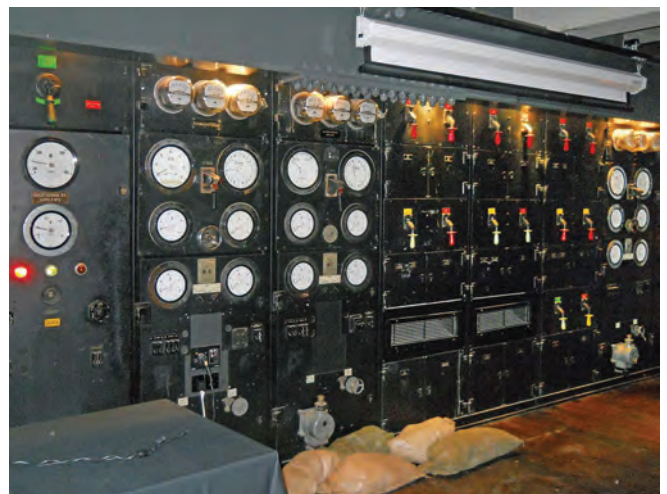
Power plant control panels. Photo Bill Ridgeway
